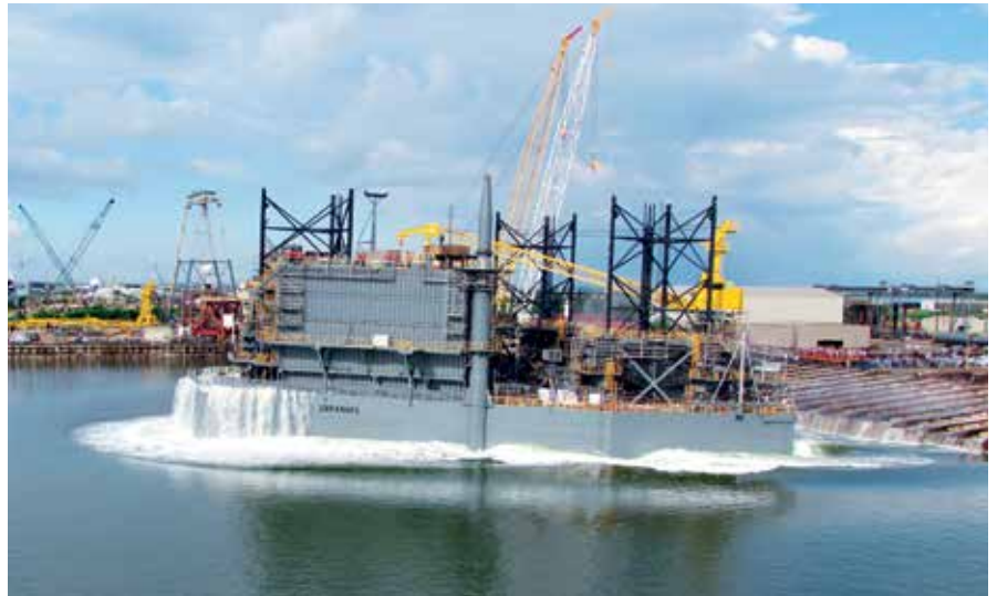
The construction of the jackup rig, Uxpanapa, reached a significant milestone with the launching of the hull into the sea
